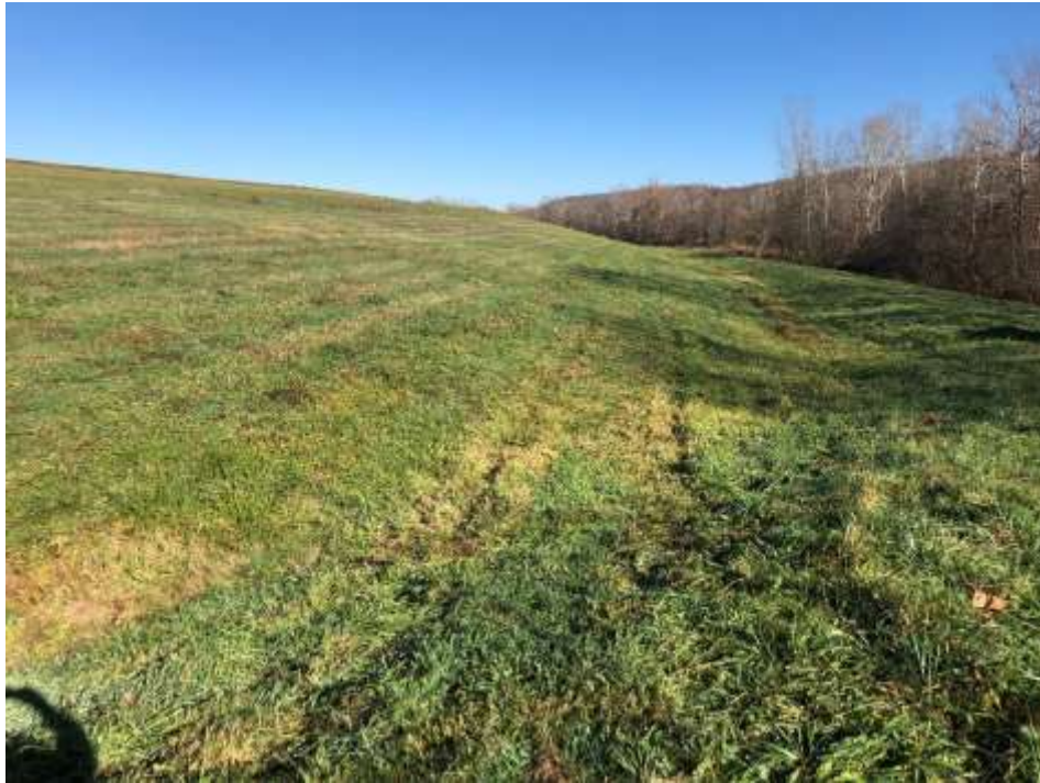
Photograph 43: East non-contact stormwater channel is clear of obstructions. East final cover lower slope is well vegetated and mowed annually. No evidence of animal burrows, erosion, or stability issues.
