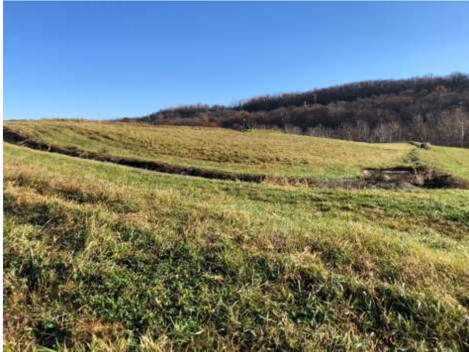
Photograph 19: South non-contact stormwater bench is clear of obstructions. South final cover upper slope is well vegetated and mowed annually. No evidence of animal burrows, erosion, or stability issues.
