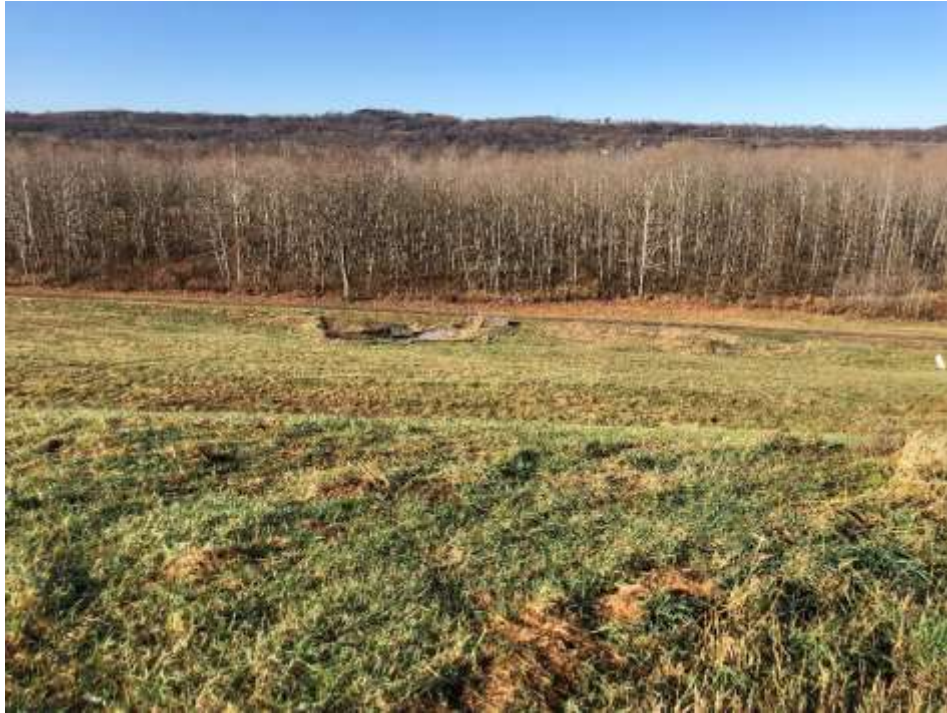
Photograph 7: Stage 4 west slope is well vegetated and mowed annually. No evidence of animal burrows, erosion, or stability issues on the vegetated slopes.
