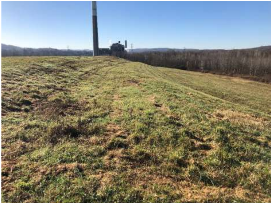
Photograph 8: Stage 4 west slope is well vegetated and mowed annually. No evidence of animal burrows, erosion, or stability issues.
