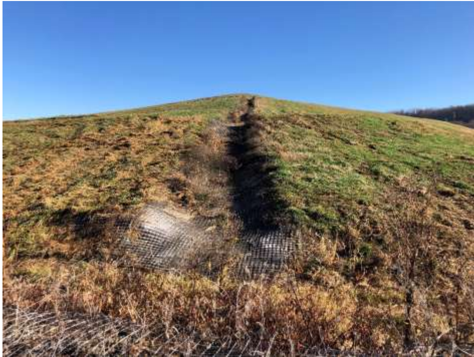
Photograph 27: Non-contact stormwater downchute is clear of obstructions. Gabion energy dissipator is installed at the junction with the stormwater perimeter ditch.
