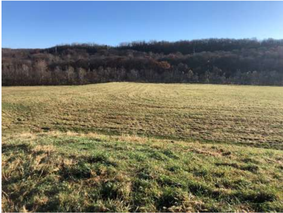
Photograph 3: Stage 6 final cover is well vegetated and mowed annually. No evidence of animal burrows, erosion, or stability issues.
