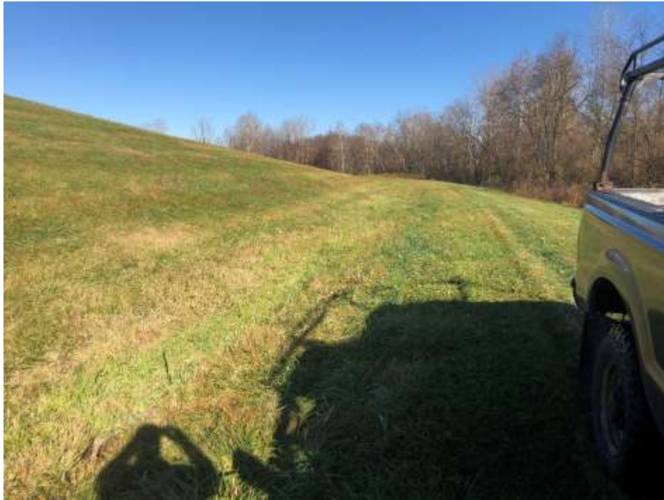
Photograph 41: East non-contact stormwater channel is clear of obstructions. East final cover lower slope is well vegetated and mowed annually. No evidence of animal burrows, erosion, or stability issues.
